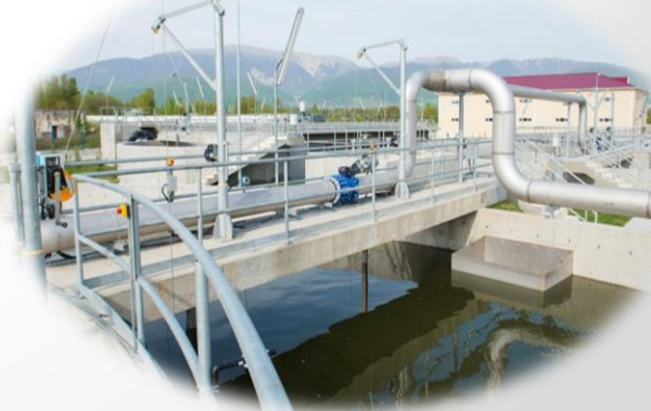
Water treatment projects for 2 regions with World Bank cooperation
